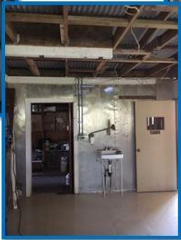
Refrigerator & freezer area
